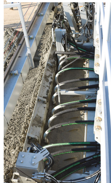
View of the grout box from operator's platform. Shown with spread auger, strike off, grout box auger, and tamper bar
