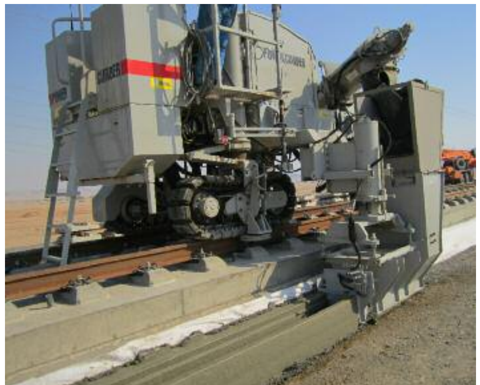
High-speed rail application in Saudi Arabia using custom rail attachments to pour a utilities trough.
