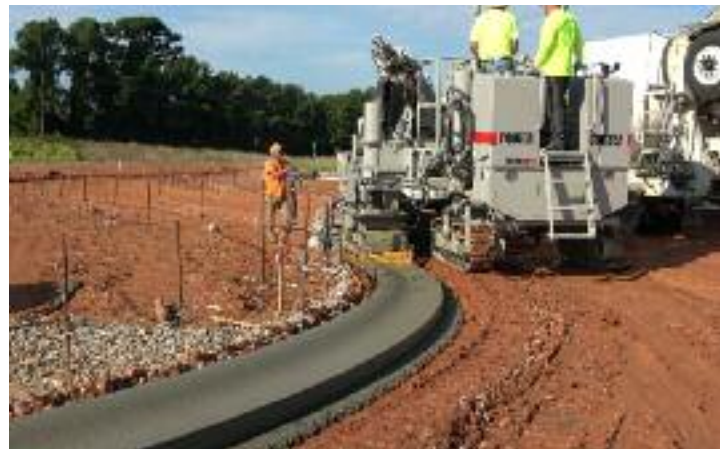
The rear post on the 5700-D-MAX can be returned to its standard position for pouring curb and gutter.
