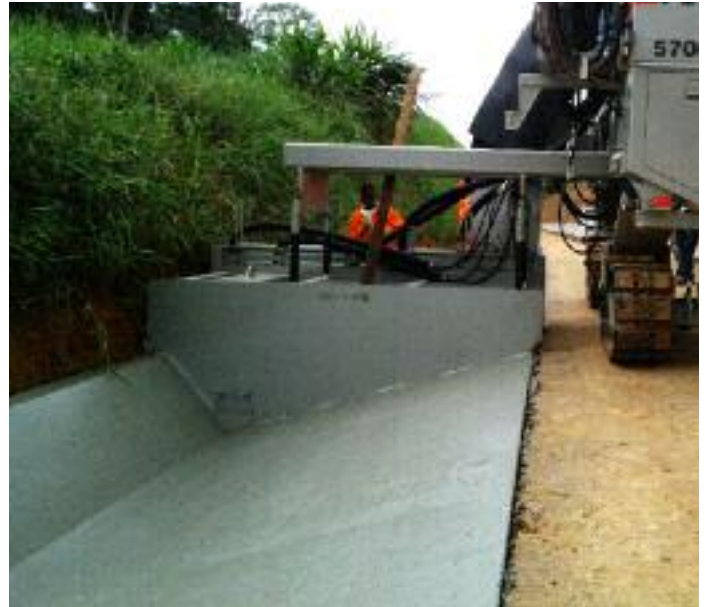
V-Ditch in Equatorial Guinea, 7' (2.2m) wide and 18" (.45m) deep, poured adjacent to pavement.
