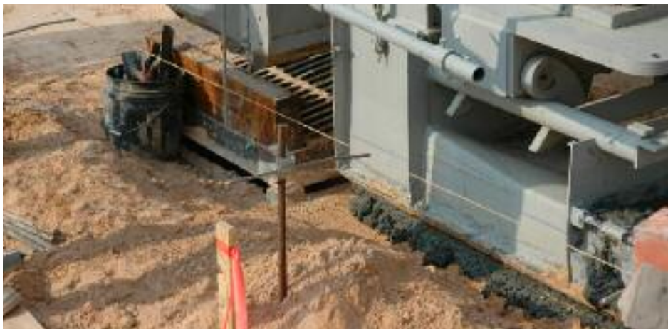
Trimmer lifting over catch basin to pour the curb as closely as possible.
