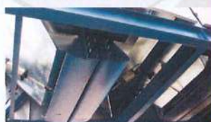
Hopper & radial doors, insulated and heated
